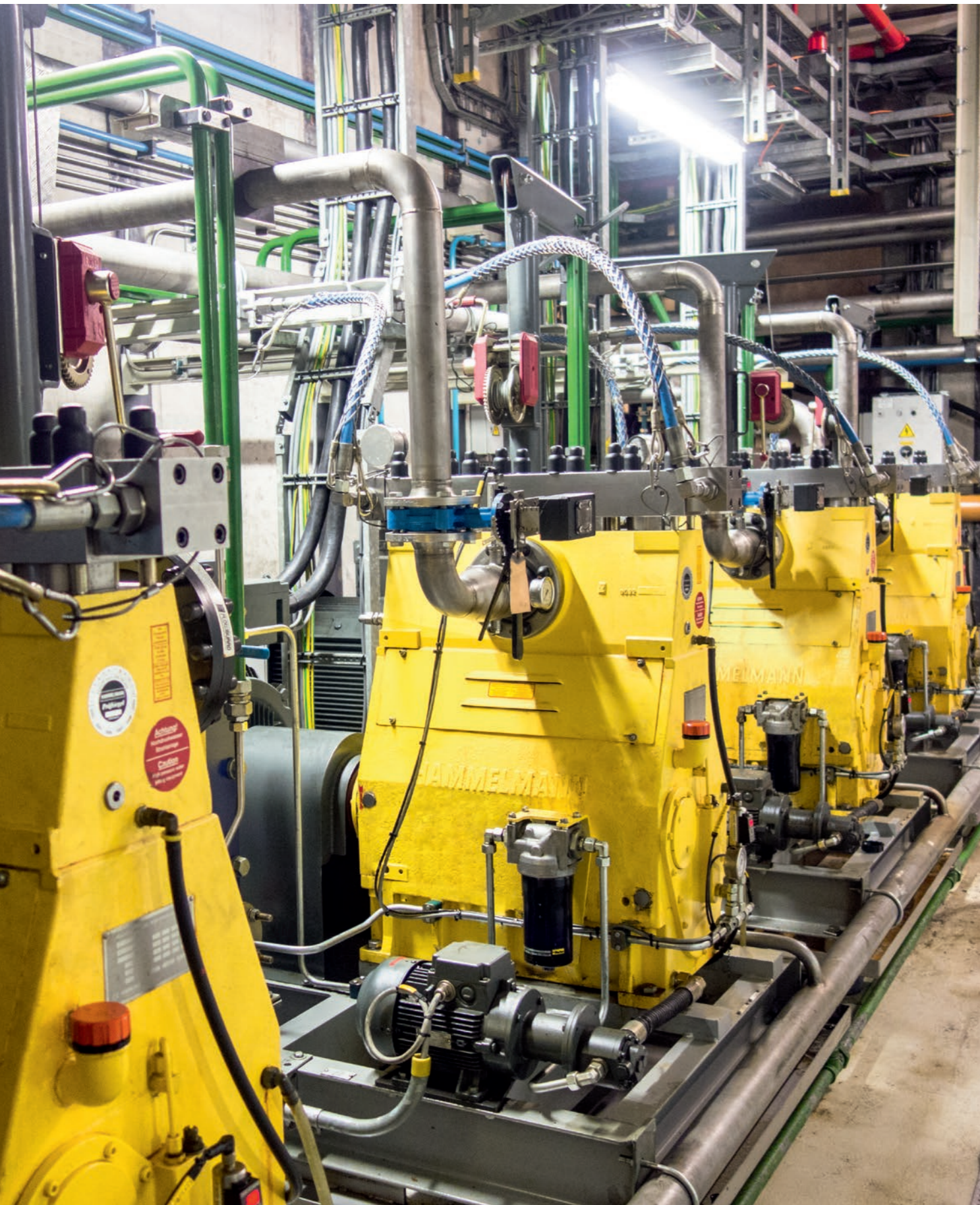
High pressure pumps in the aluminium industry. Above in operation since 2009 with an average of 5000 operating hours per year.
